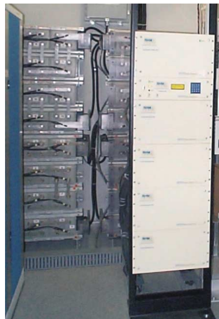
Fig. 8. 100 A BHM TM system in wireless telecommunication tower application.
